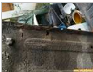
3 => Pare-boue : corrosion perforante
